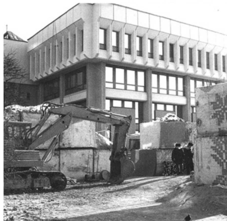
War-like sights by the building of the Supreme Council in Vilnius, Lithuania.
